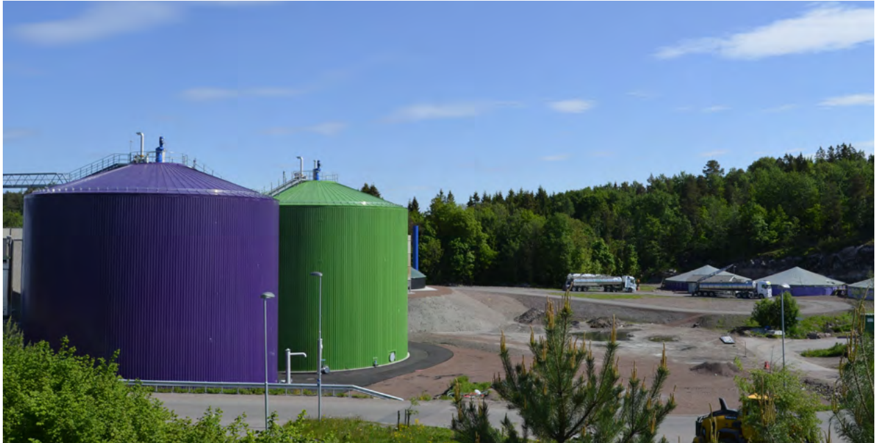
Greve Biogass is increasing production of climate-friendly biogas at the colourful facility in Tønsberg (Photo: Greve Biogass).
